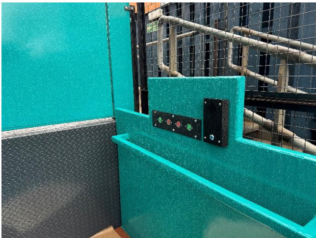
(A close-up of the vertical platform lift control buttons)
